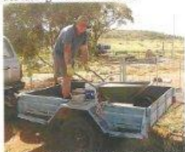
A batch of concrete from 'On the Spot ready mixed concrete' about to be unloaded by 'operator', Ian Husband.
